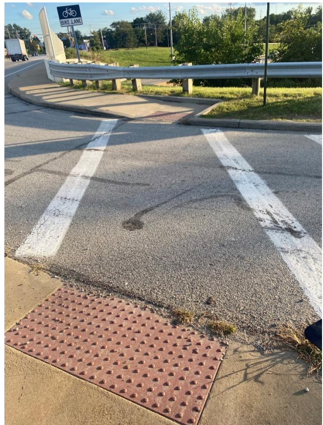
Curb cuts and tactile markers not aligned to safely assist a visually-impaired pedestrian
