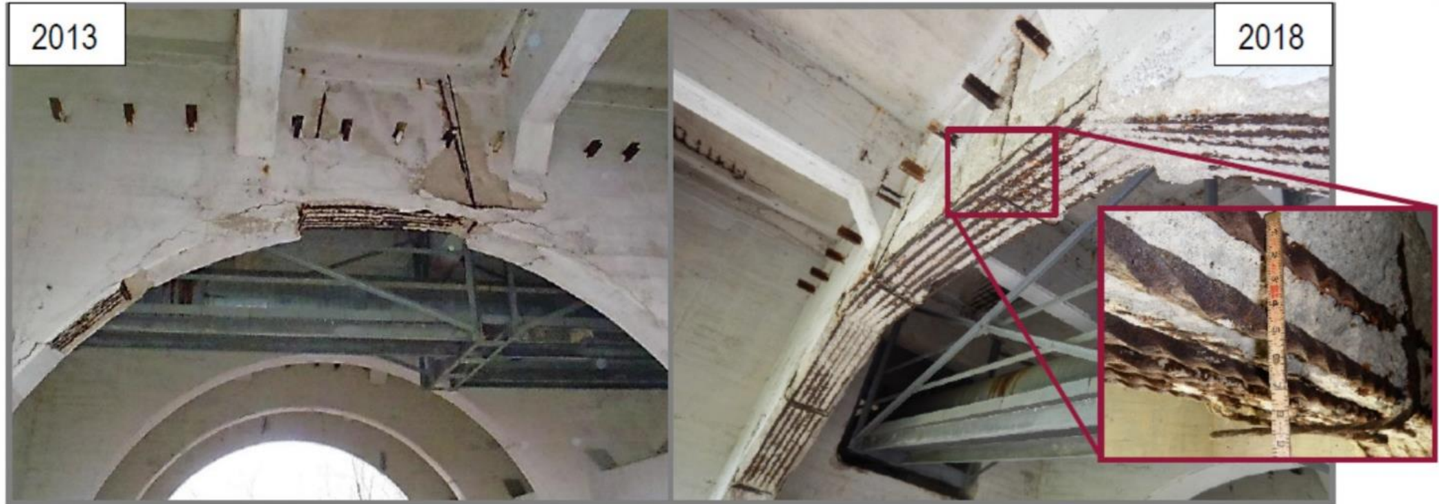
Deterioration to the underside of the arch
